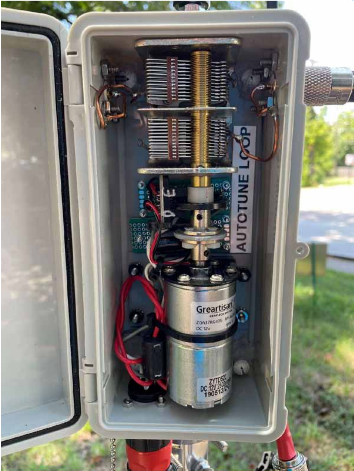
Inside view of Motor/Capacitor Box, note insulated motor coupler.
